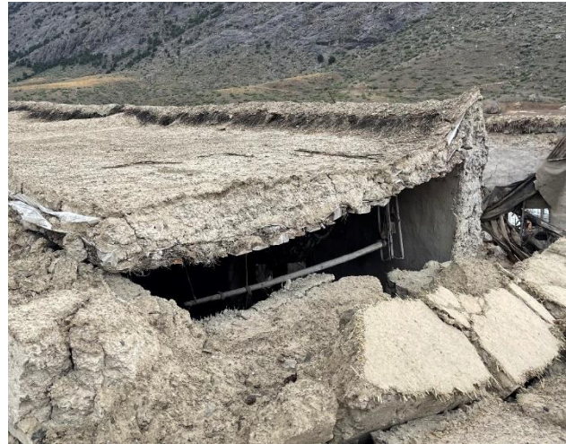
Figure 2-13. Failed section of multilayered roof.
