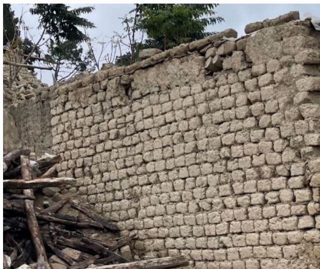
Figure 2-16 Example of poor mortar joints, poor rain protection and poor course work.
