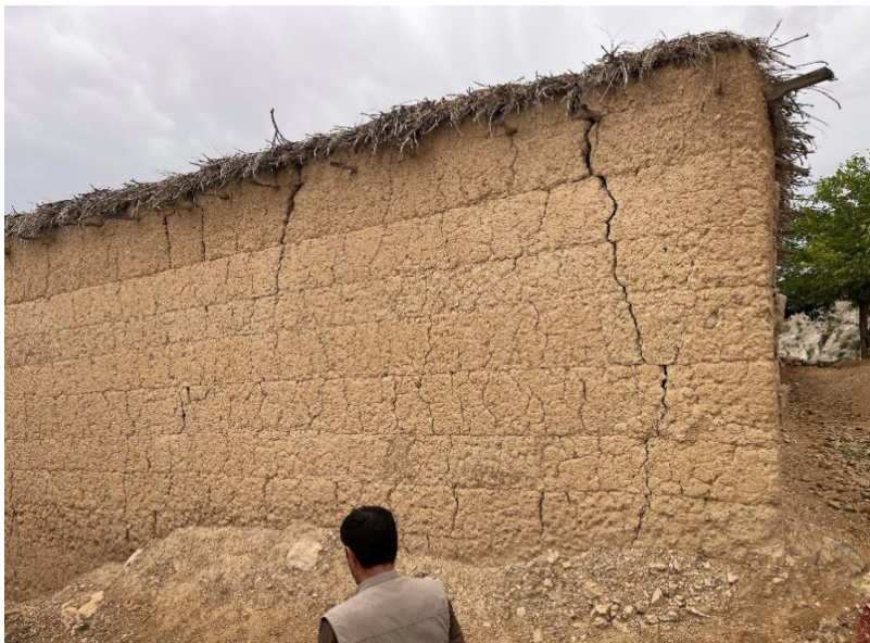
Figure 2-11 Example of commonly observed partial corner detachment.
