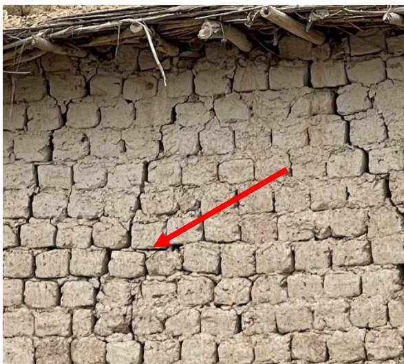
Figure 2-17. Example of insufficient coursing.
