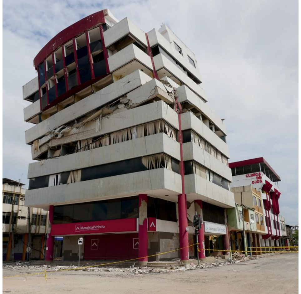
Severe damage to buildings in Portoviejo, Ecuador following the April earthquake.
