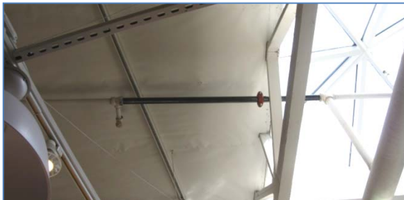
Sprinkler lines and heads impacting structural members or other suspended equipment caused pipe breakage and water damage.
