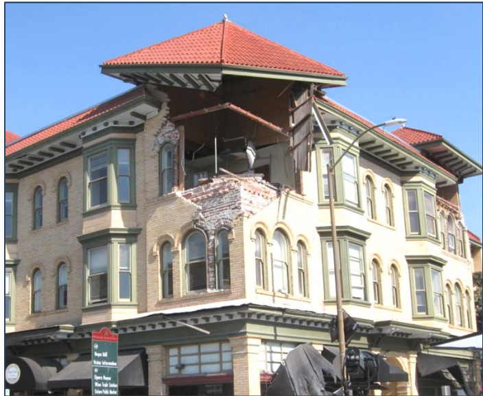
Damaged retrofitted unreinforced masonry building (URM) at 2nd and Brown Streets, downtown Napa.
