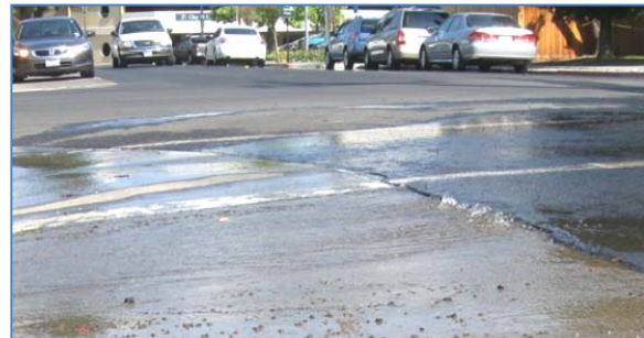
Water bubbling up through downtown pavement - one of 120 water line breaks in Napa.
