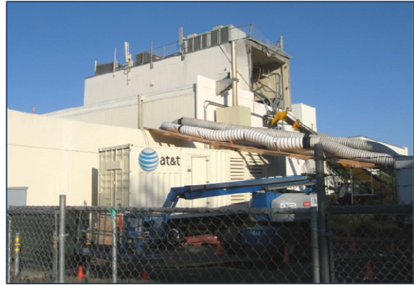
Downtown Napa AT&T building was red tagged due to rooftop equipment anchorage failure and knock-out wall panel fallout.
