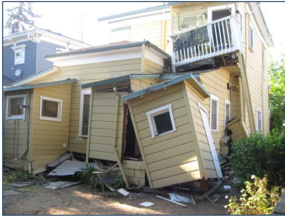
House not bolted to its foundation slid and dropped.
