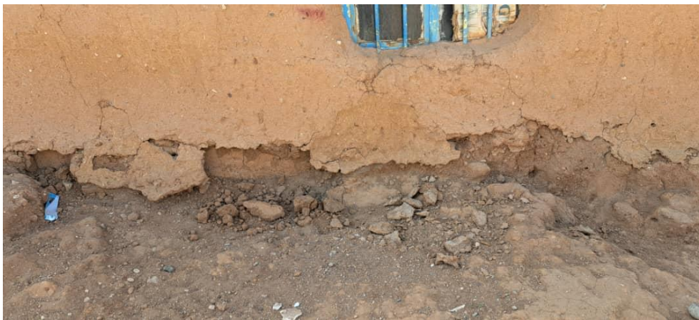
Figure 2 No rock foundation and rock stem wall.
